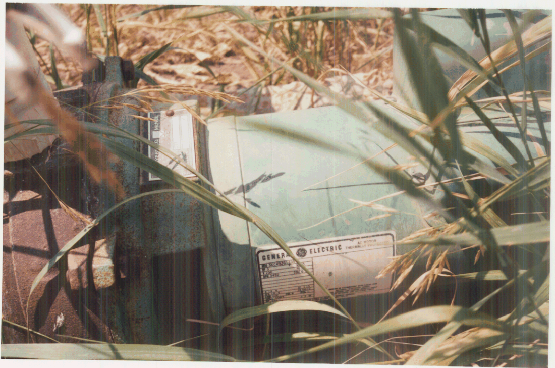
Looking @ Pump. Pump info in FE Notes.
