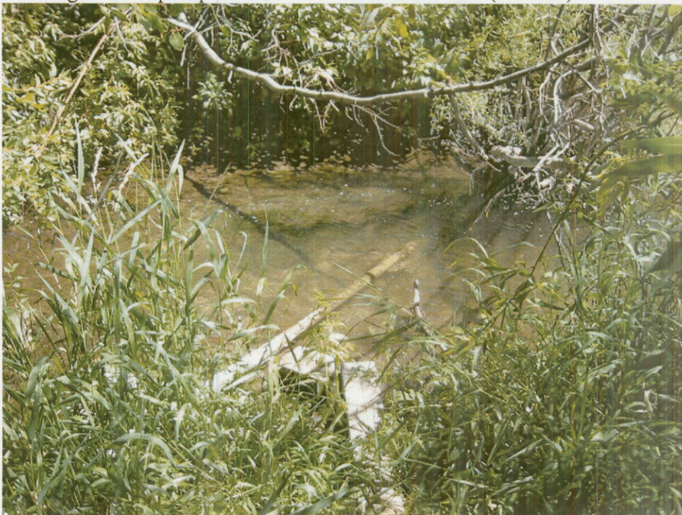
Looking East at white PVC intake line and POD (saxton).
