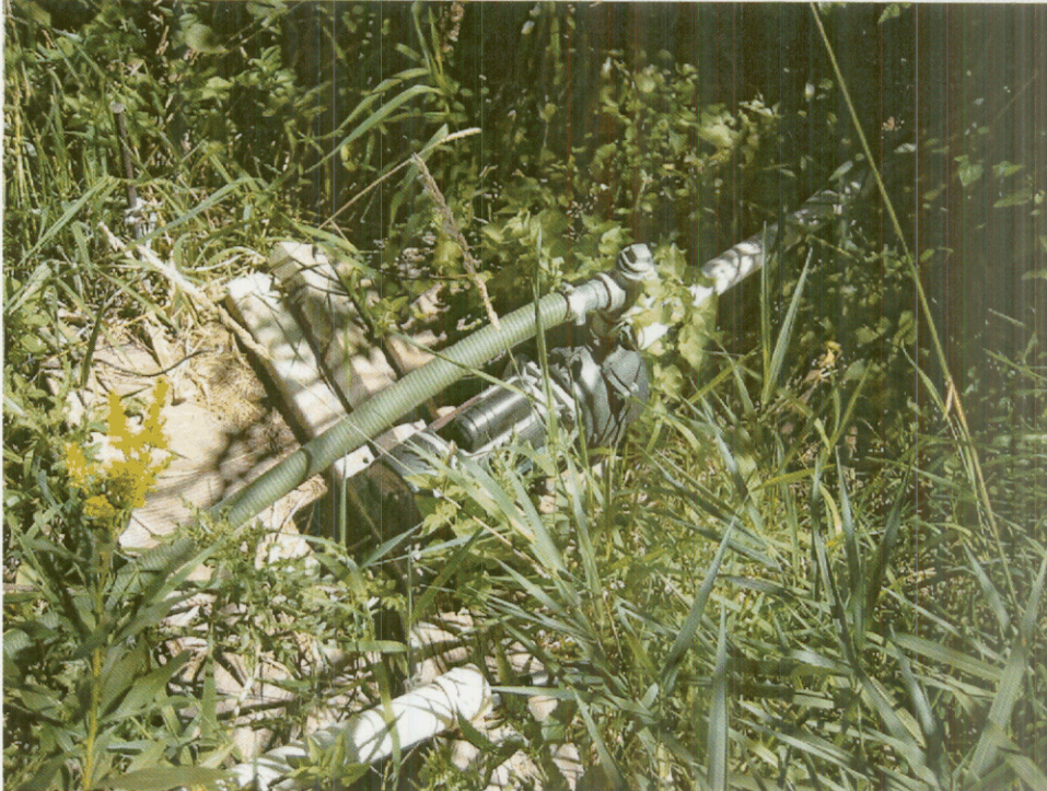
Looking at POD pump. White PVC is the intake line (csaxton).
