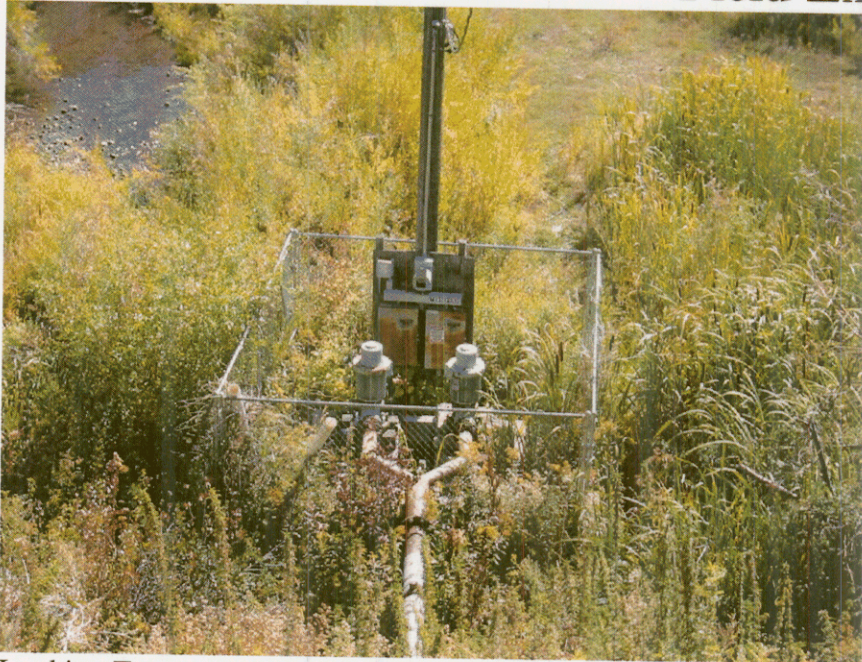
Looking East at two pumps that feed into a common system. Mink Creek in Background.
