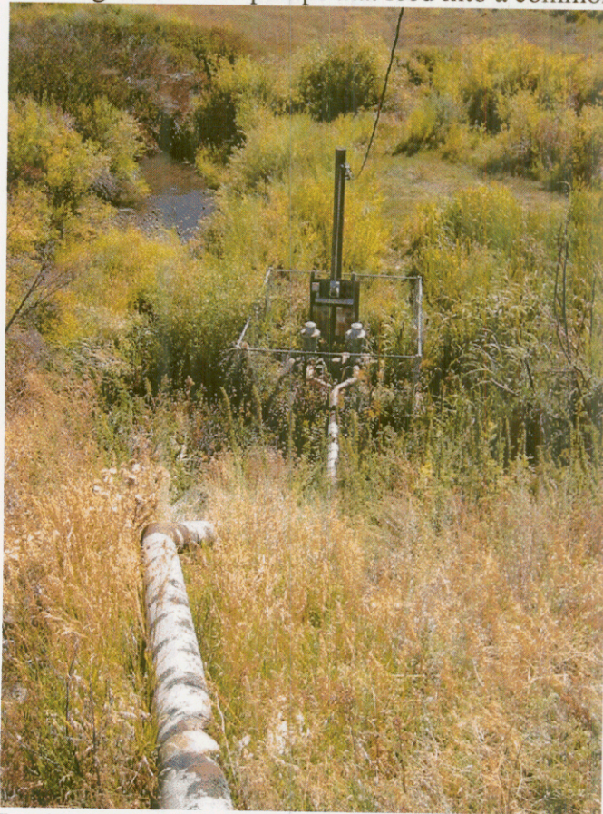
Looking East at two pumps that feed into a common system. Mink Creek in background.
