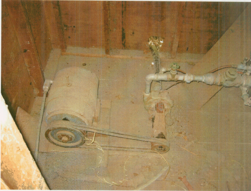
Looking inside POD pumphouse. Pump info: Make = Crane; SN = 448039; HP = ? (csaxton).
