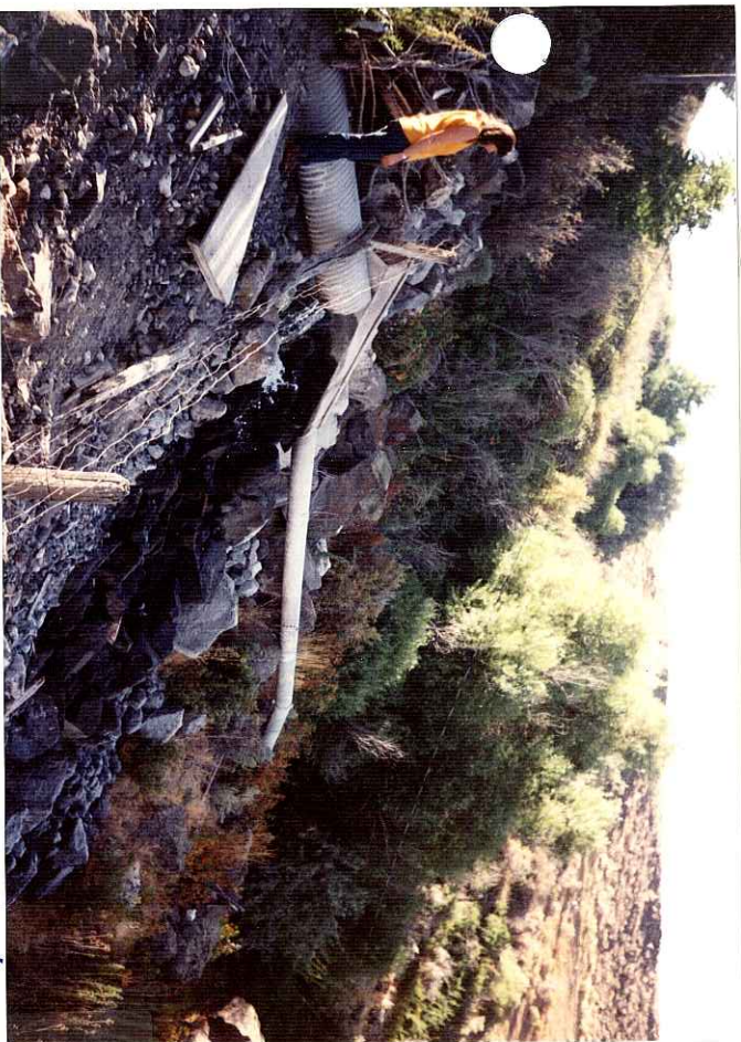
WATER SINKS INTO ROCKS, RETURNS TO BILINGSLEY CREEK PIPELINE DISCONNECTED
