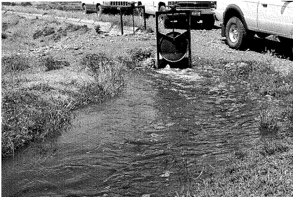
Photo 9. Discharge from pump into earthen ditch. Flow can also be turned into the concrete slip-form ditch in the background (which was dry today).
