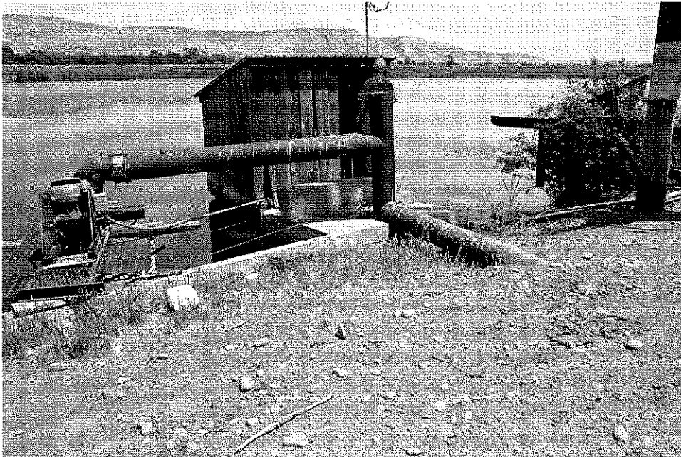
Photo 8. Unnamed slough diversion system includes 25-hp pump into earthen ditch and/or concrete slip-form ditch.
