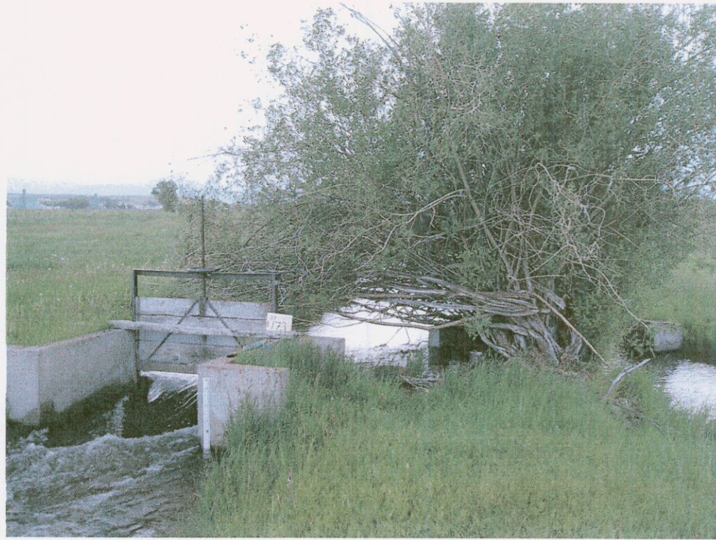
Blair Ditch headgate diverts out of Spring Creek.
