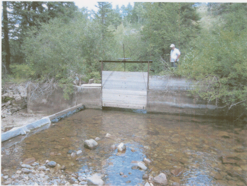
Garden Irrigation System (Darby Creek) Todd Canal headgate in Wyoming
