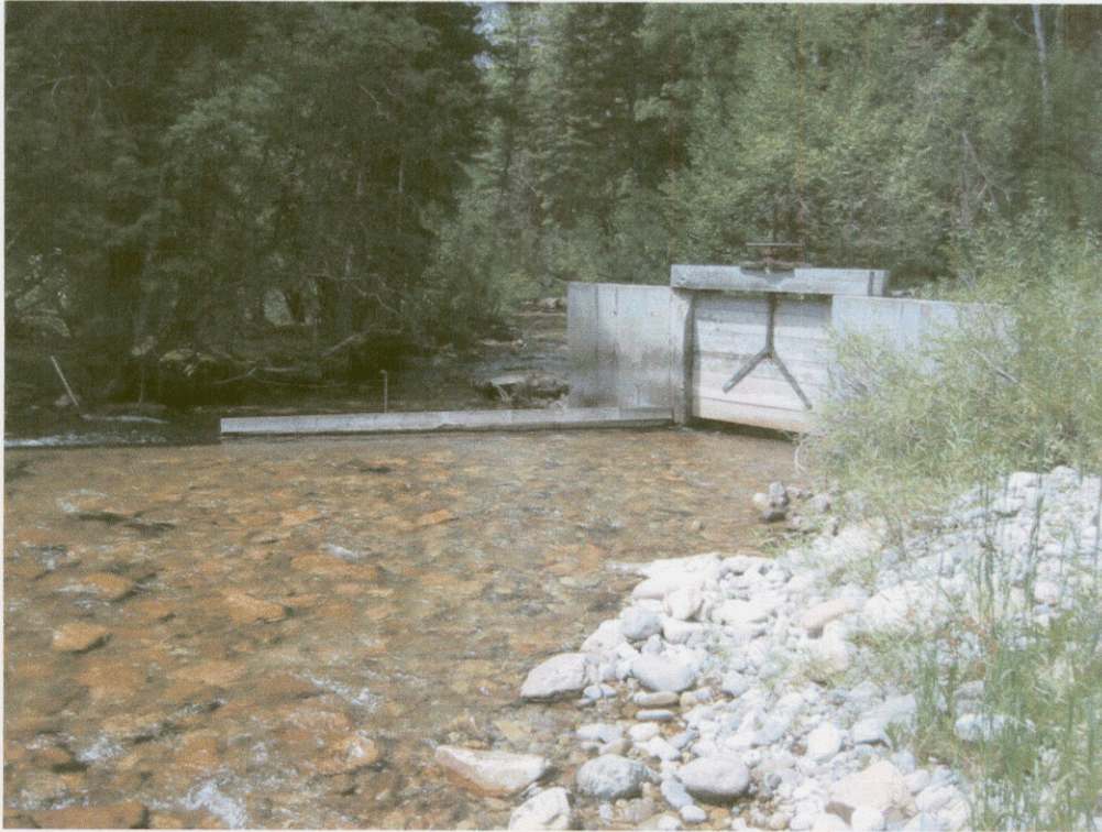
Garden Irrigation System (Larby Creek) Hill Canal headgate in Wyoming
