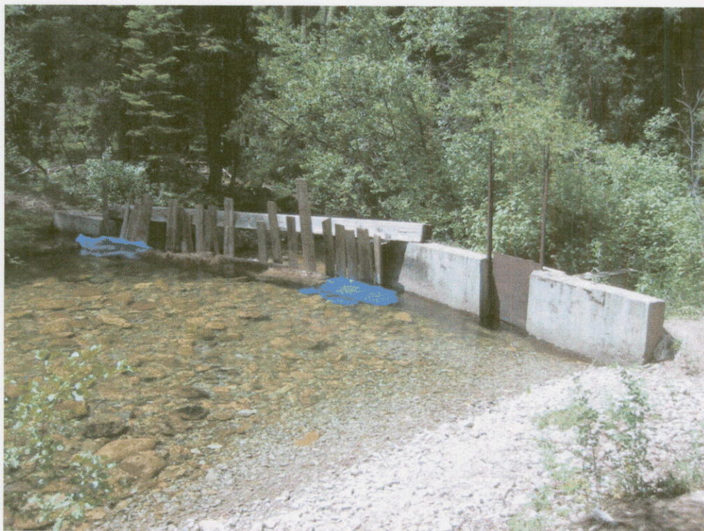
Garden Irrigation System (Darby Creek) Winger Canal headgate in Wyoming
