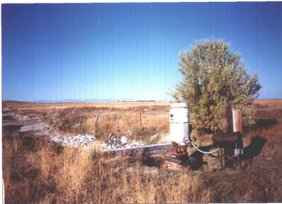
Pump #1, Photo #1. 100 horsepower motor nameplate.
