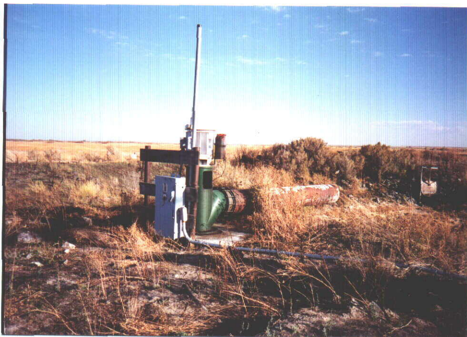
Pump #3, photo #3. 100 horsepower motor nameplate.
