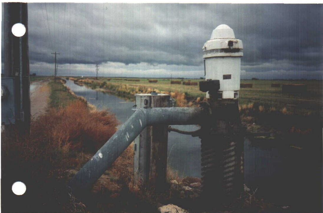
Photo #1-6 10/5/94 Looking SE FROM 15' NW OF P.D. SHOWING PUMP USING WASTE DITCH AS SOURCE, MAIN LINE GOES UNDERGROUND TO THE NORTH.
