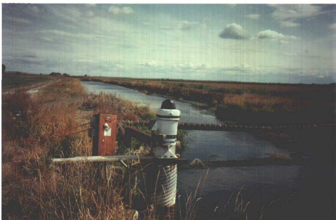
PHOTO #1-7 10/6/94 LOOKING SE FROM N BANK OF DRAIN DITCH SHOWING PUMP #2 FEEDING MAINLINE GOING BOTH N AND S ACROSS THE DRAIN DITCH, 1/4 MILE FROM JEFFERSON CANAL.
