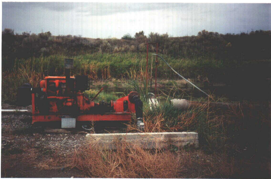
PHOTO 1-4 10/5/94 LOOKING SE FROM 15' NW OF THE DIESEL PUMP POD SHOWING THE WASTE DITCH SOURCE. THE MAINLINE GOES UNDERGROUND TO THE NORTH
