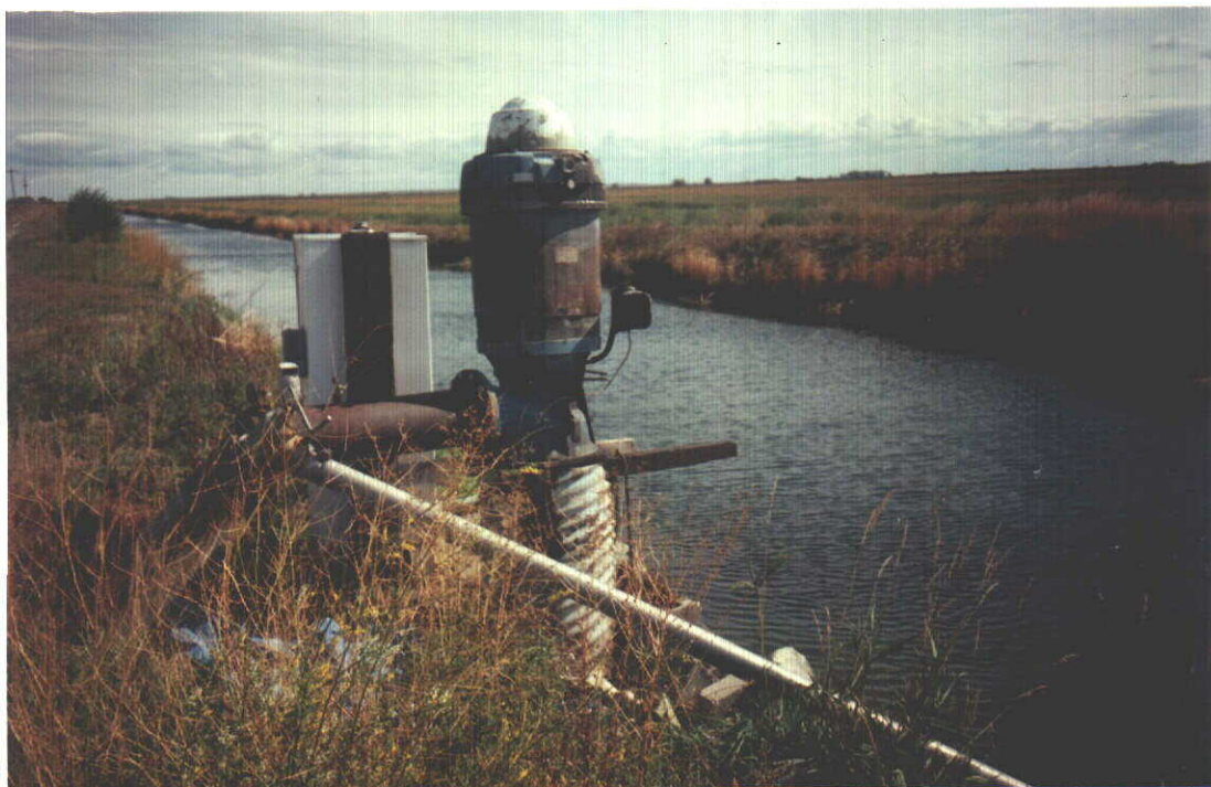
PHOTO #1-8 10/6/94 LOOKING SE FROM N BANK OF DRAIN DITCH SHOWING PUMP #3 FEEDING UNDERGROUND MAINLINE GOING TO THE N. 1/2 MILE FROM JEFFERSON CANAL.
