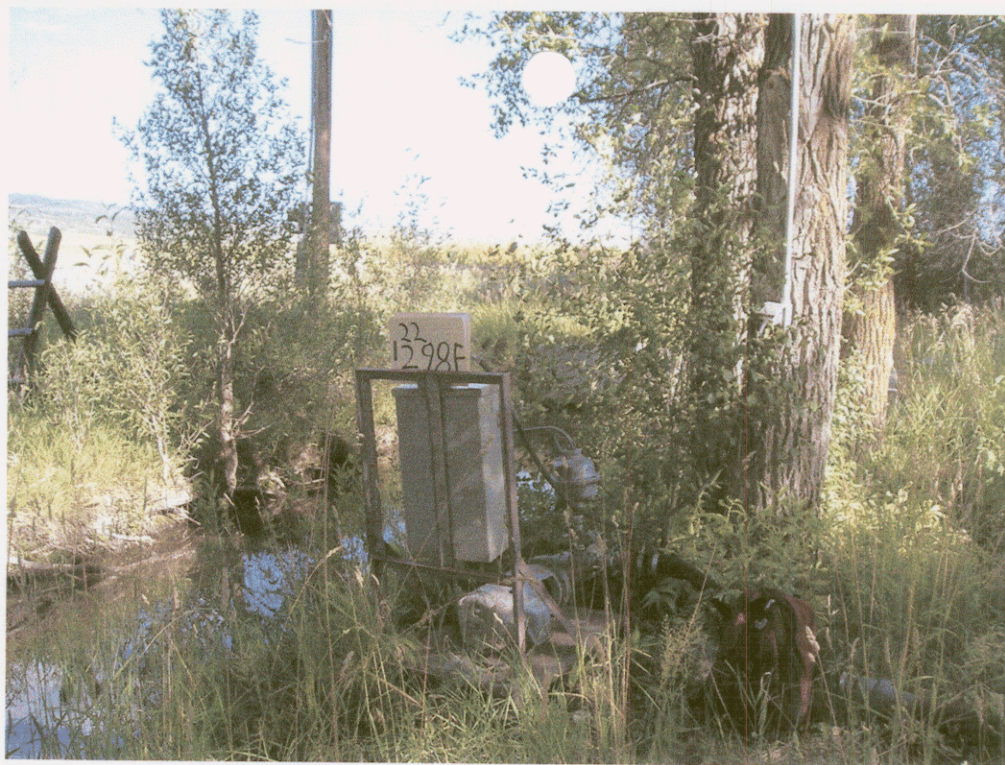
Tom Knight pump on Horseshoe Creek. Tag on electric panel.
