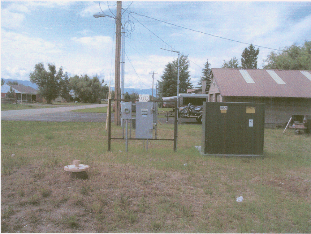
Driggs City well on 5 th East & Ross Ave.
