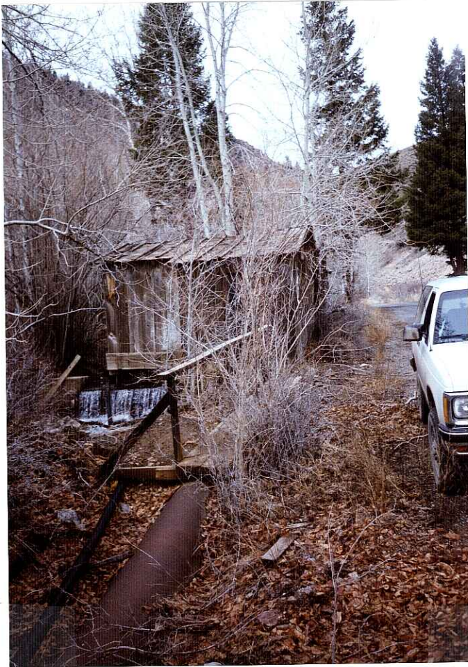
↗ PENSTOCK ↖ DOMESTIC USE LINE TO CRAWFORD
