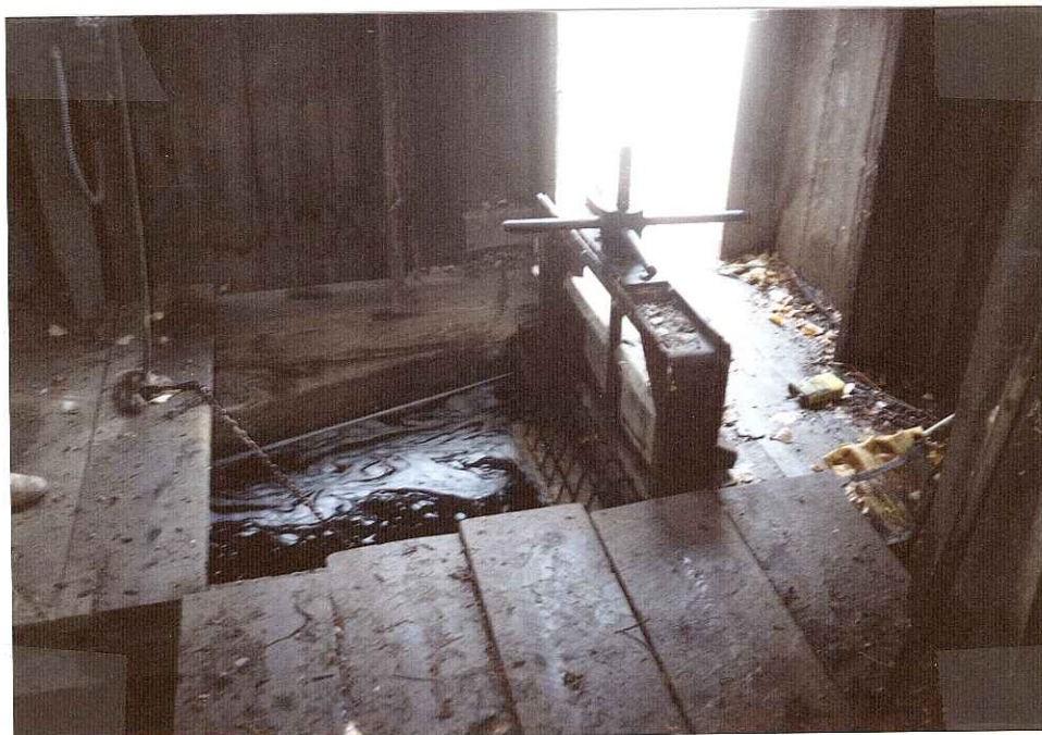
CONTROL GATE © PENSTOCK
