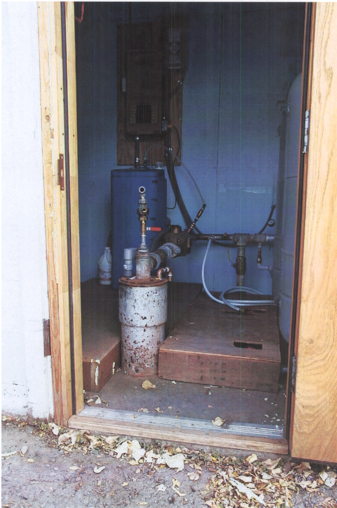
10/7/2003 Well + pressure tanks. 5HP
