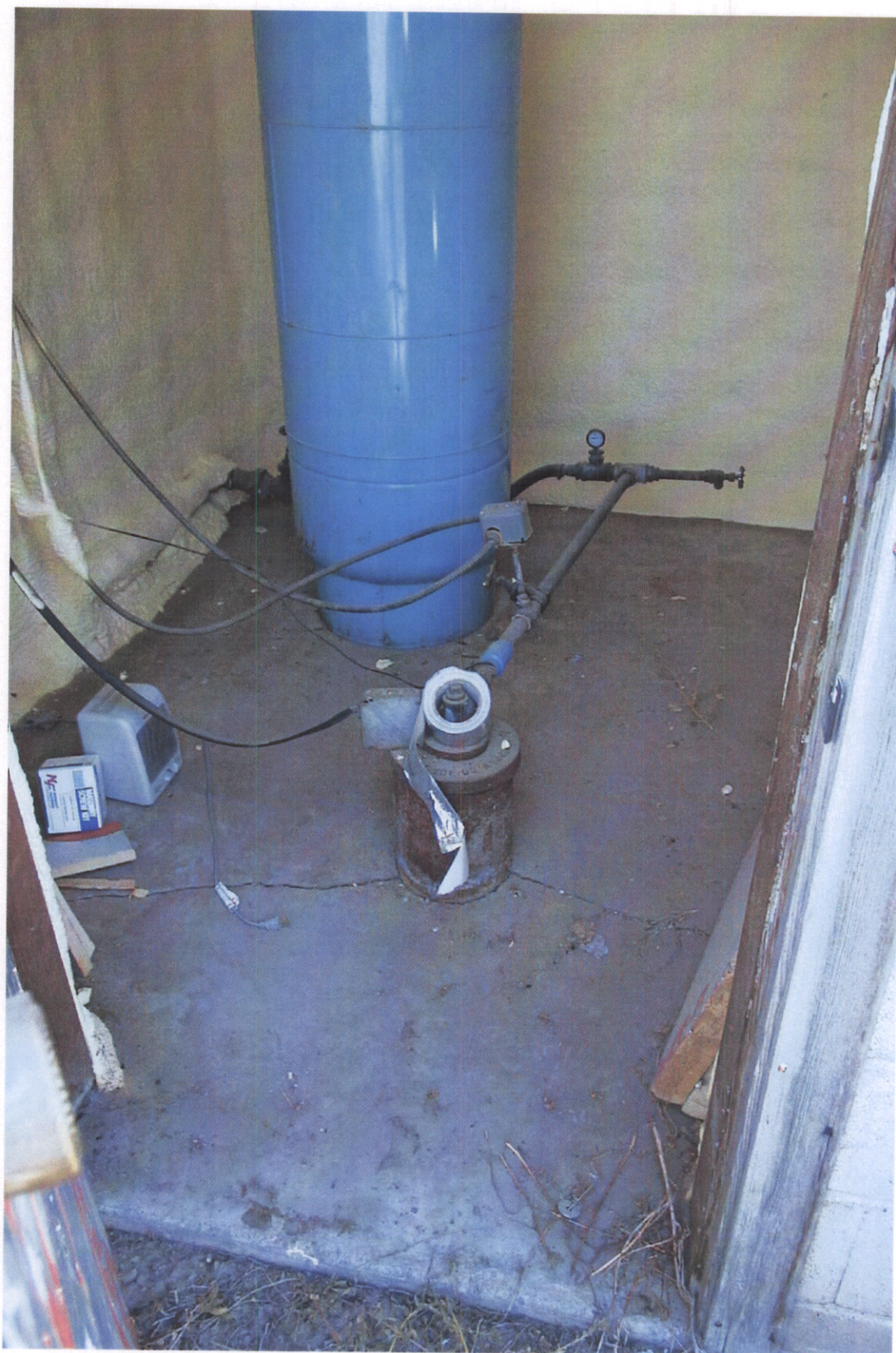
9/30/2003 WELL, PUMP, + PRESSURE TANK
