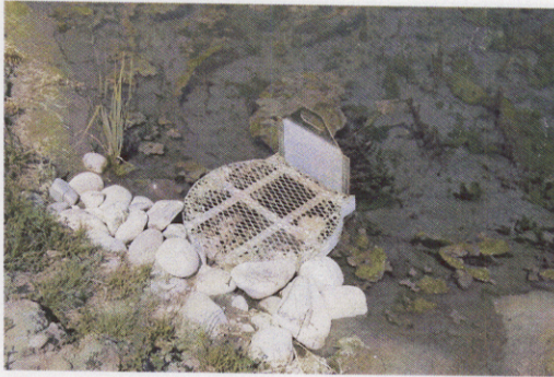
Slide gate in pond.
