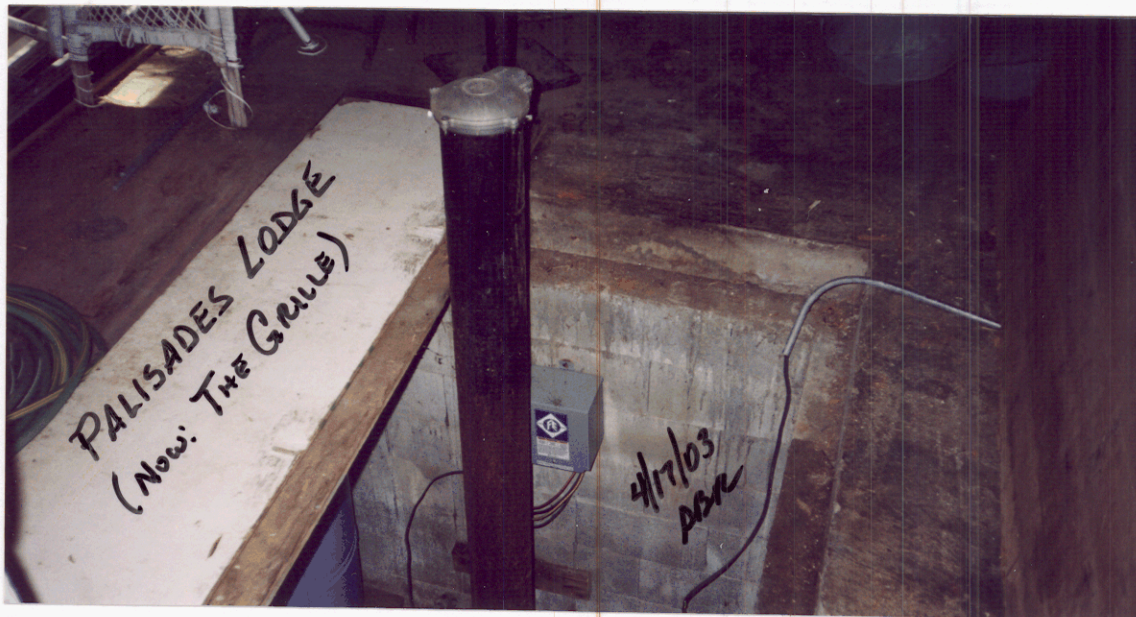
SHOWS CASING INSIDE BLOCK WELL HOUSE.
