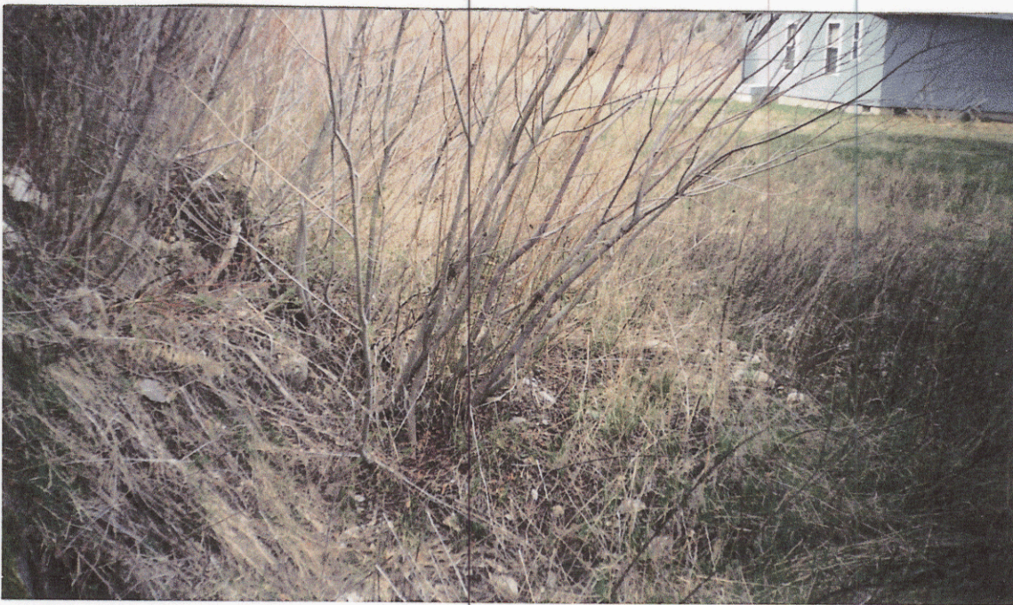
Photo 2. Shows A PLACE BEHIND THE BLOCKAGE OFF THE CREEK. OBVIOUSLY THERE HAS BEEN NO MAINTENANCE AND NO DELIVERY FOR A LONG TIME.
