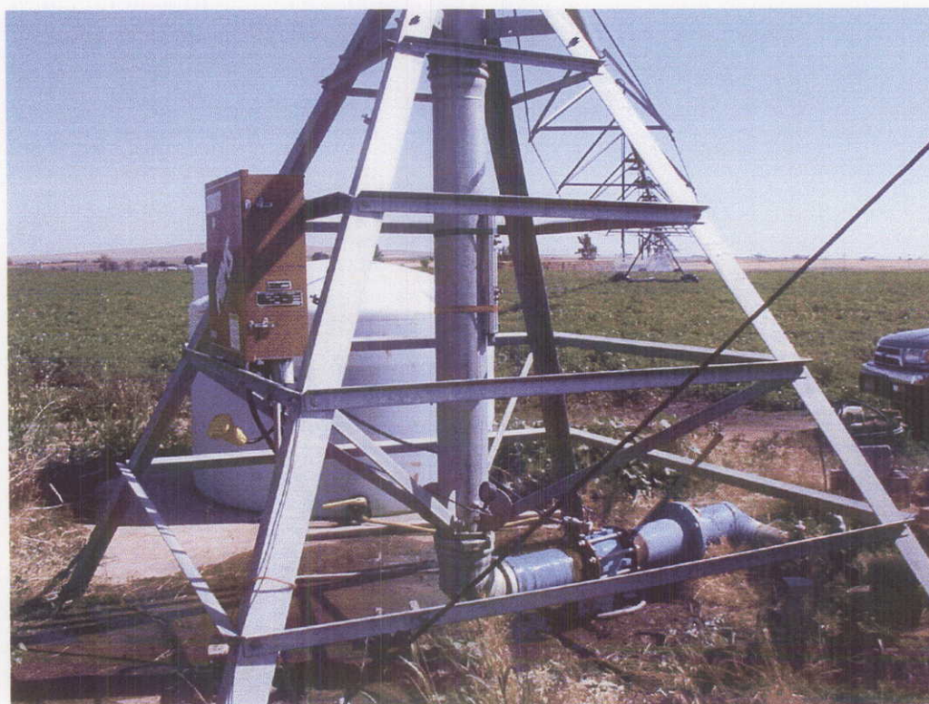
East pivot flow measurement
