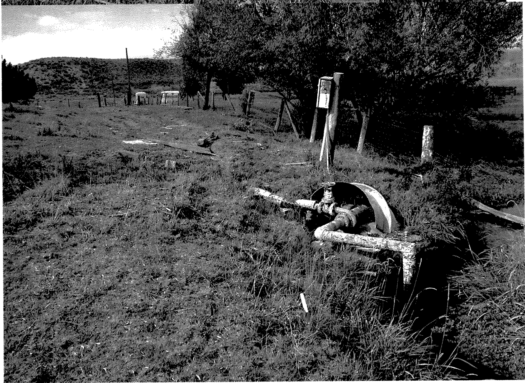
10/2001 - P02 7.5 hp pump to DAVE CARLSON sprinklers and open discharge
