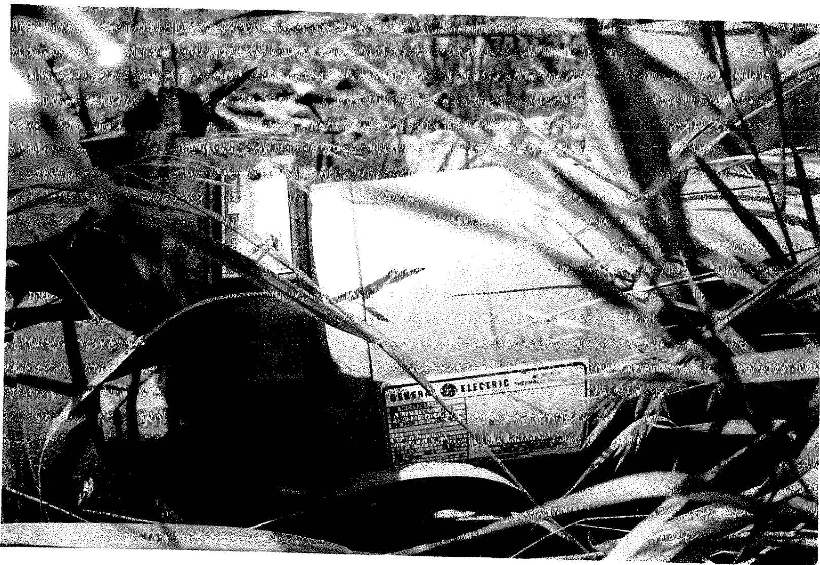
looking @ Pump. Pump info in FE Notes.
