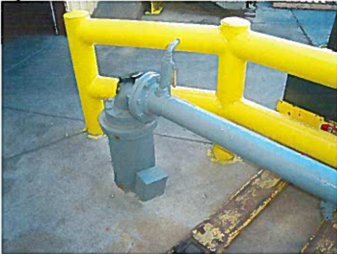
Figure 2: Wire that appears to have been cut to Small well
